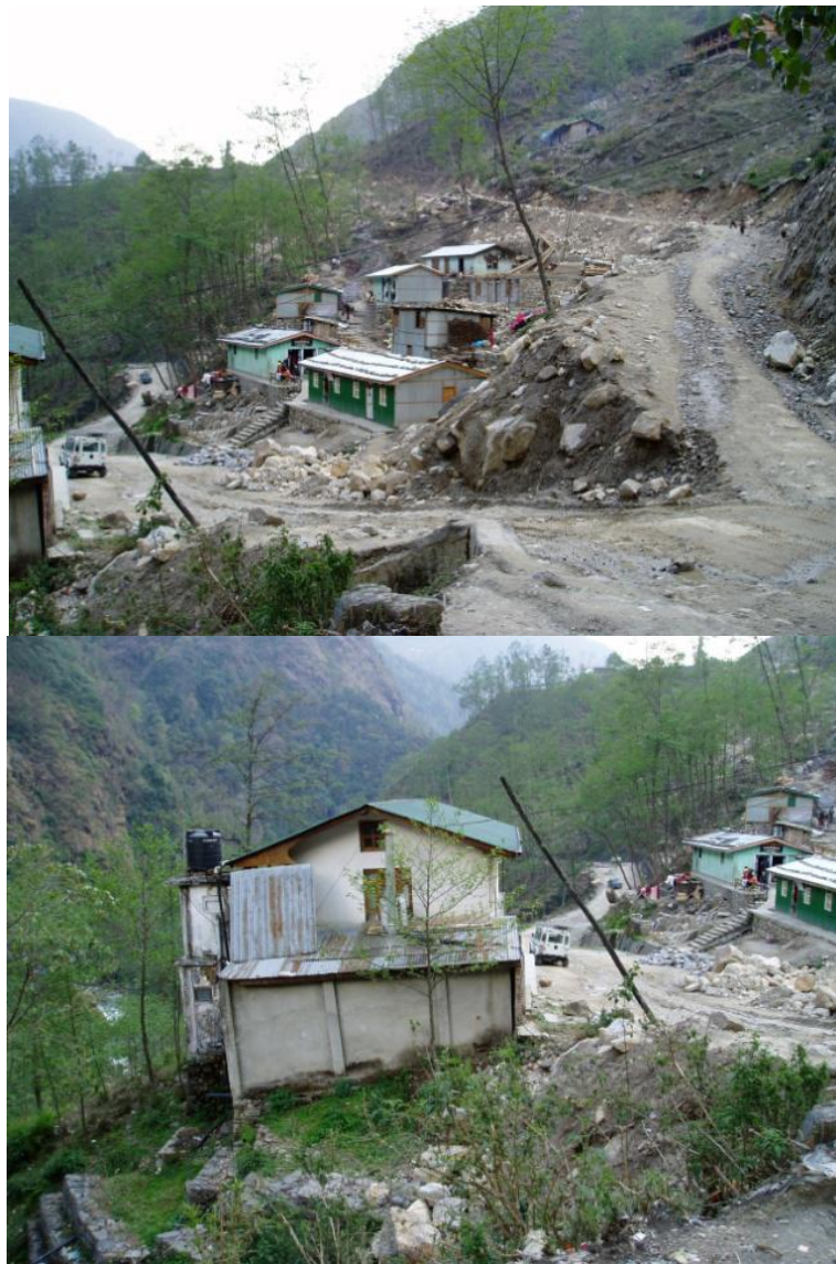
Figure 4.19 The roadside settlement of Kodari. Inclining trees, marked changes in the level of the road and cracks in the Eco Hotel (bottom photograph) are indicators of continuous slope movement.
